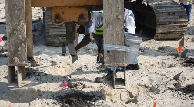
The so-called "anchor-plate" is wrapped around the end of the strip to prevent the strip from being pulled up after pushed into the weak soil.
