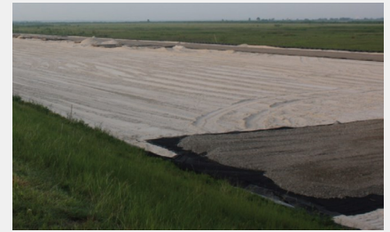
Non-woven geotextile layer is installed to separate the sand and crushed stone layers.
