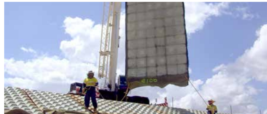
Enka-Fix is strong enough to lift the concrete mats in the air
