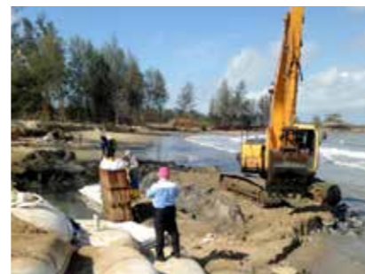
Enka-G-Bag is filled with in situ sand which avoids the transport of rock or fill material.
