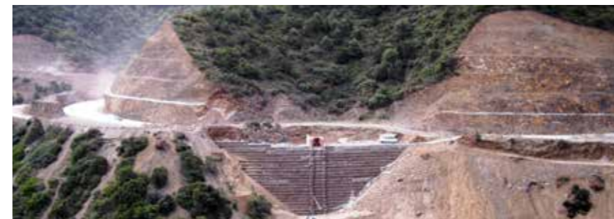
Enkagrid retaining solution minimised the load on top of the existing slopes
