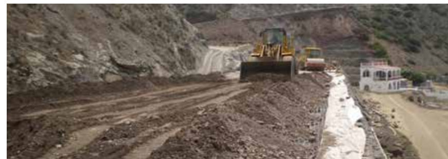
Levelling/compaction of the filling, gabions being used as well as temporary formwork, Enka-Tex pending layer on the gabions
