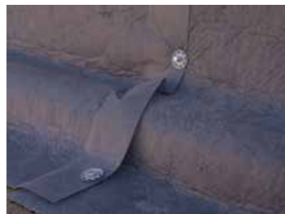
At the bottom, Enkadrain is covering the pipe, no need of additional gravel material
