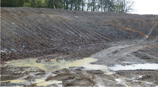
Cut and removal of rock base to accommodate the main retention pond as a part of golf course irrigation system
